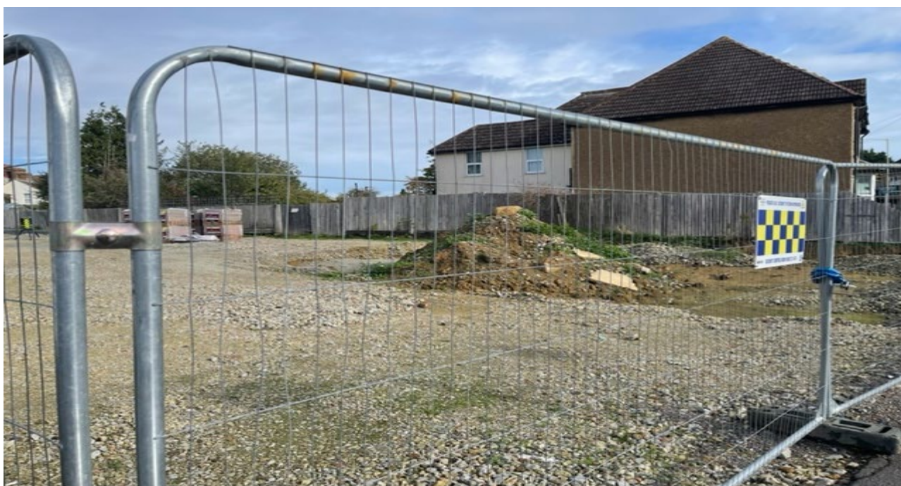
Figure 3: Photo showing the flank elevation of the dwelling. The adjacent car park (under construction) in the foreground
